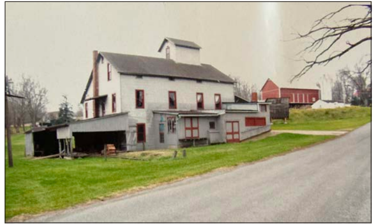
KISTER MILL is located in Millbrook, Ohio. This photo was taken before restoration. It now has new siding and a new roof.
